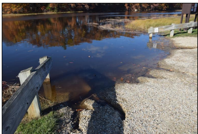
Erosion channels above boat ramp
